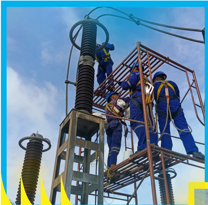
Basic & Advanced Assessment Main Trafo
