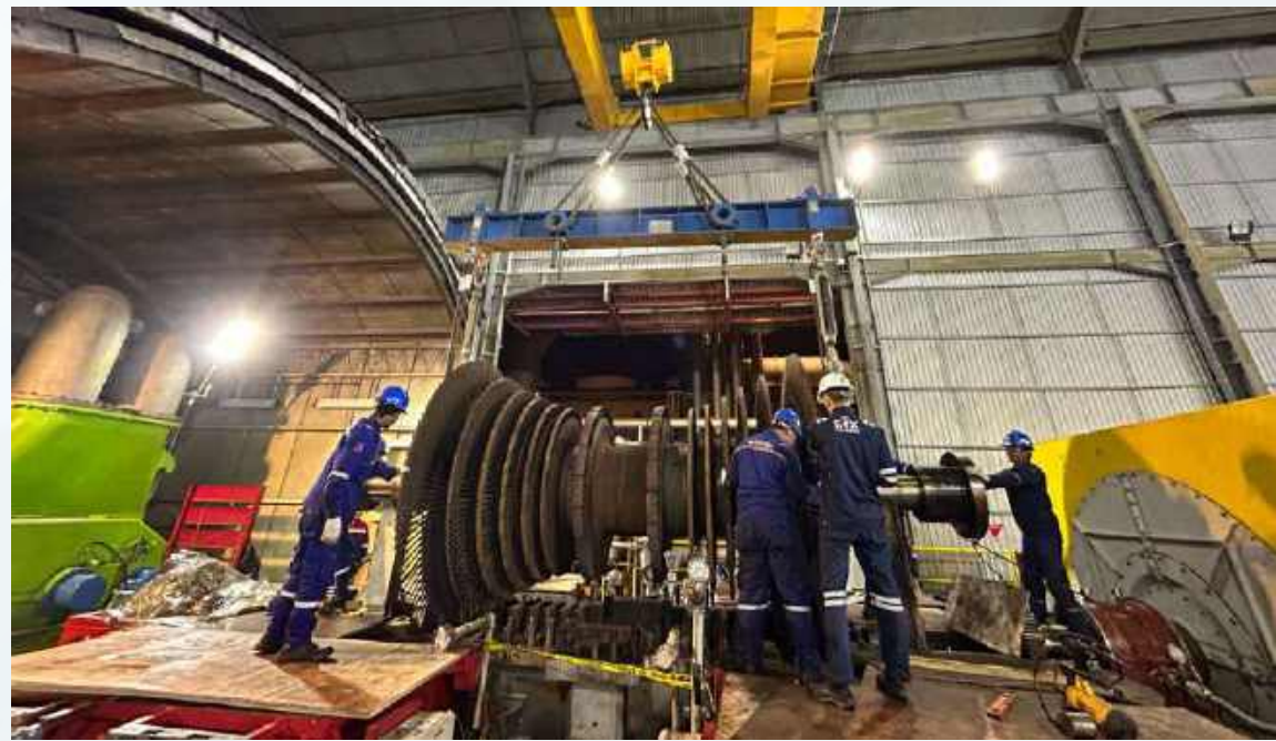
Turbine Ansaldo 60 MW Capacity
