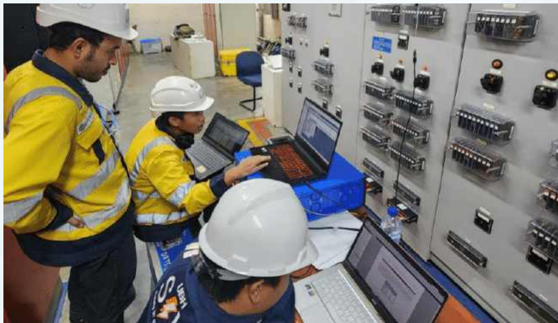
Relay Protection Verification
